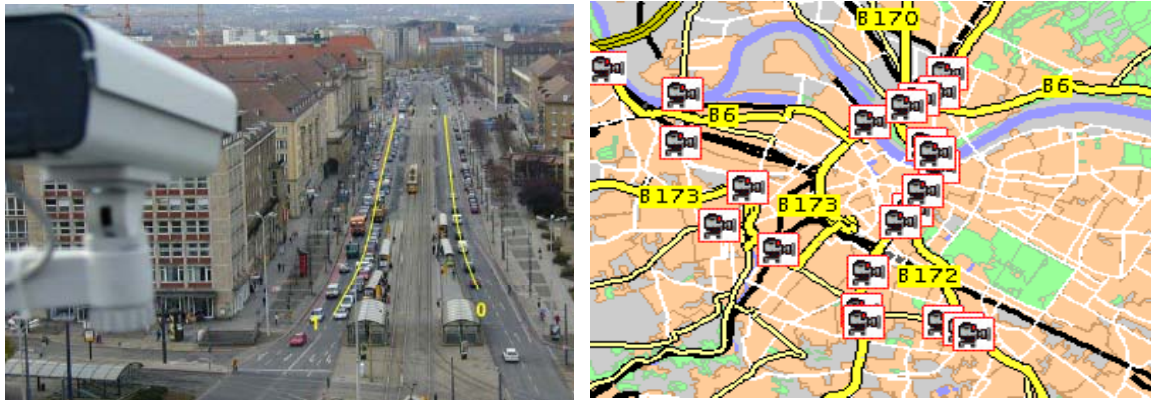
Figure 9 Video cameras installed on the most critical road's nodes are used to monitor the traffic condition.
