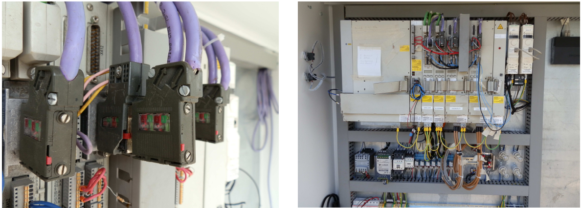
Fig. 8-9 Power electronics components assembled on generator and connections
