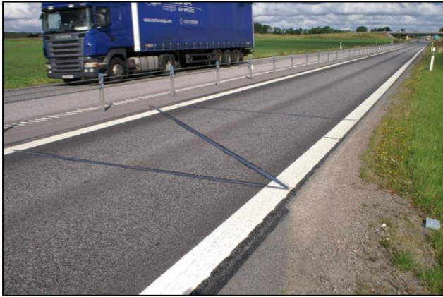
Photograph 1. Coaxial cable sensor. (Photo. Terence McGarvey)
