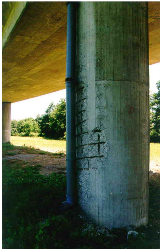
Figure 8.5: Deterioration of a column 2000
