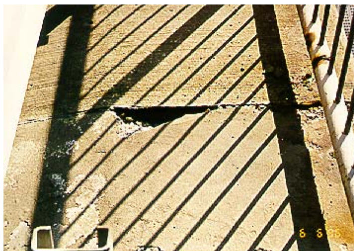
Figure 3.4: Deteriorated surface of the concrete sidewalk
