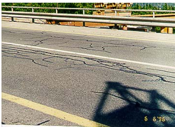
Figure 3.1: Cracks in the pavement of carriageway
