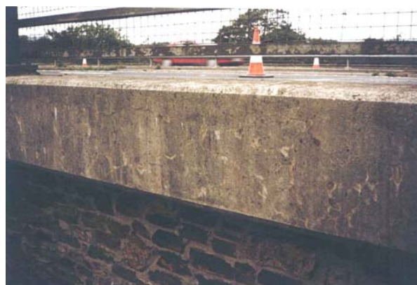
Figure 5.4: ASR affected bridge.
