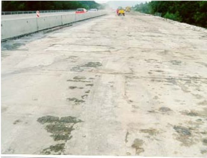
Figure 3.2: Deterioration of the bridge deck after the removal of pavement and waterproofing membrane
