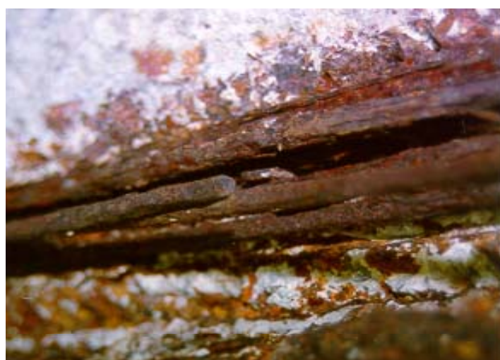
Figure 3.6: Close view of corroded tendons from the platform at major inspection
