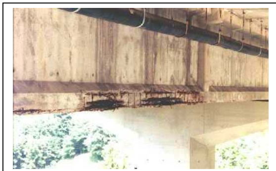
Corrosion of prestressing tendons
