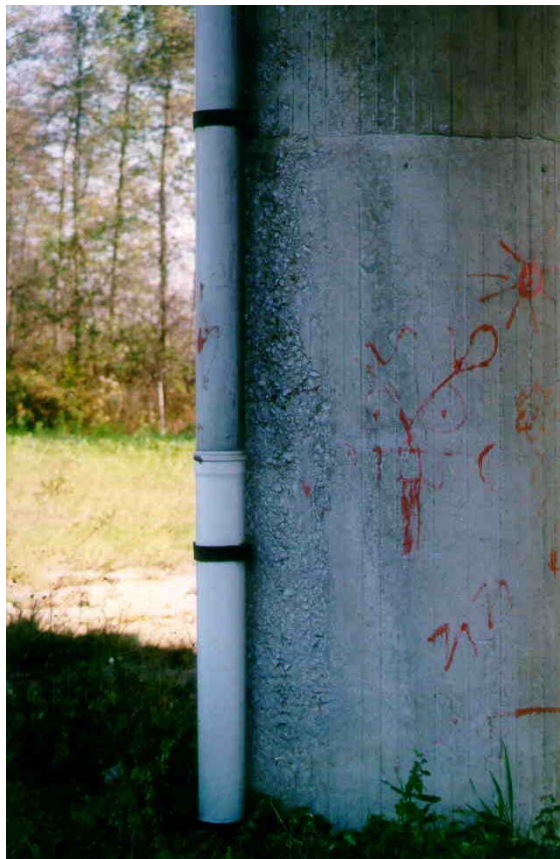
Figure 8.4: Deterioration of a column 1997
