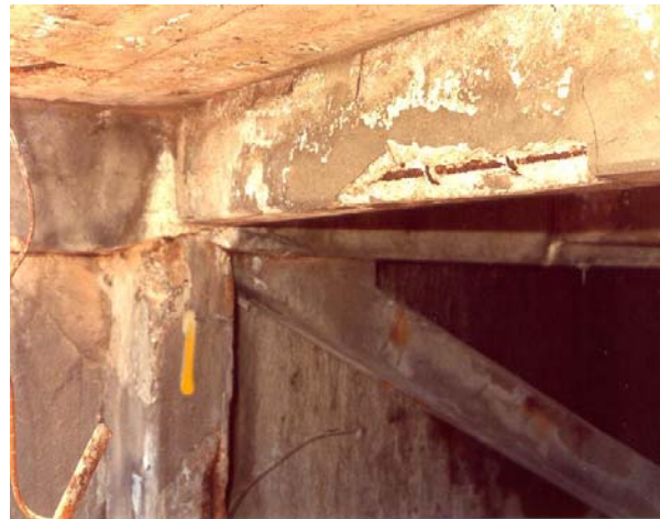
Figure 5.1: Corrosion in UK bridge.
