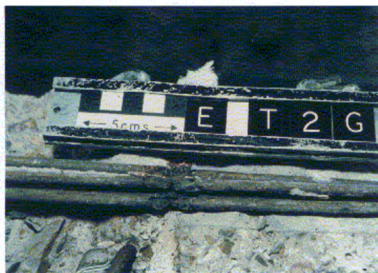
Figure 5.2: Corrosion in post-tensioning tendons.
