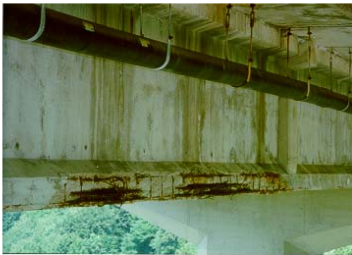
Figure 3.5: Damaged girder, access by movable platform
