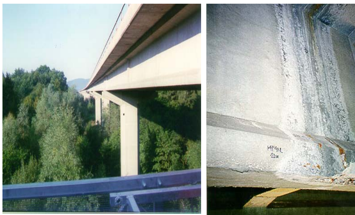
Figure 6.1: Longitudinal view on the viaduct Preloge, Slovenia. Wetting of the concrete surface of the edge beam under the damaged joint of the deck's pre-cast elements
