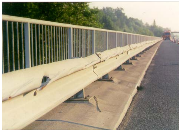
Figure 3.3: Damaged steel Guard Rail
