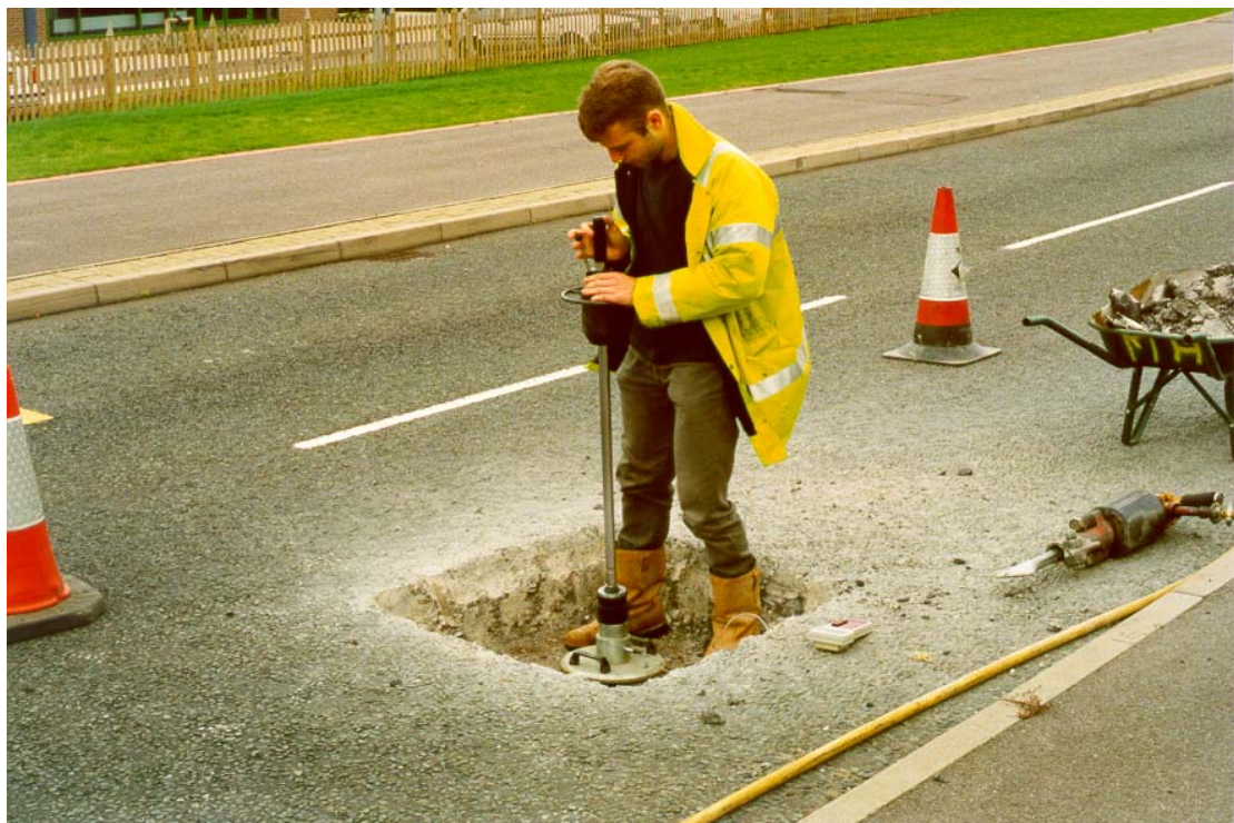
Figure 7.11 Plate bearing test (using German Dynamic Plate Bearing Test apparatus) conducted in trial pit, at Bracknell demolition rubble sub-base site
