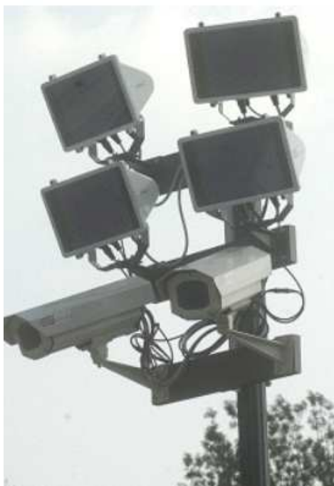
Figure 59: OCR equipment at the entrance gate [Tomassini 2001]
