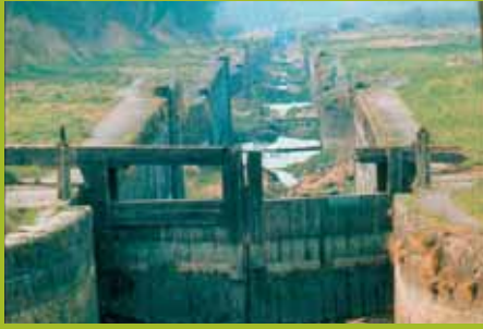
Restoration of derelict Waterways is vital
