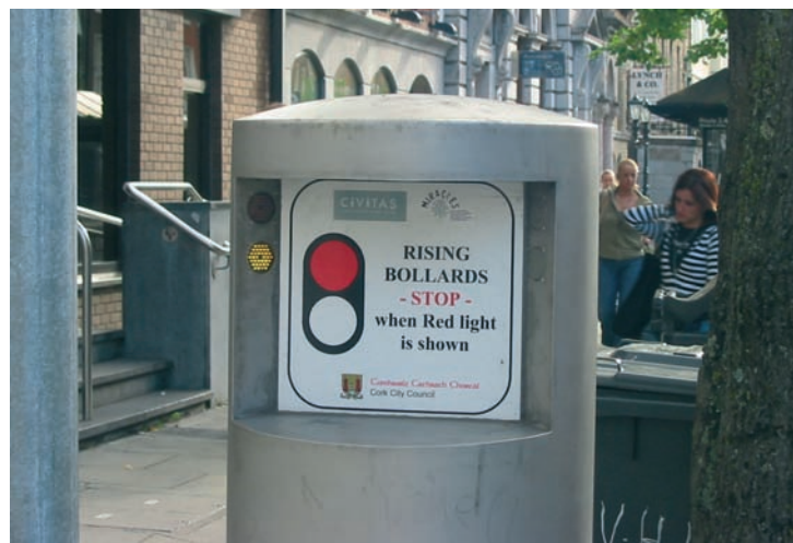
Cork: bollard control unit
