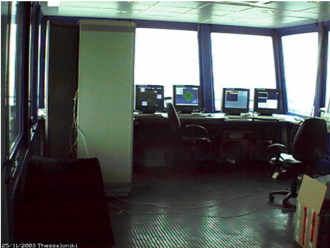
Figure 5-9: INTERVUSE Equipment Room at Thessaloniki
