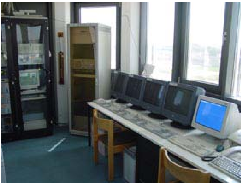
Figure 5-7: INTERVUSE Equipment Room at Mannheim
