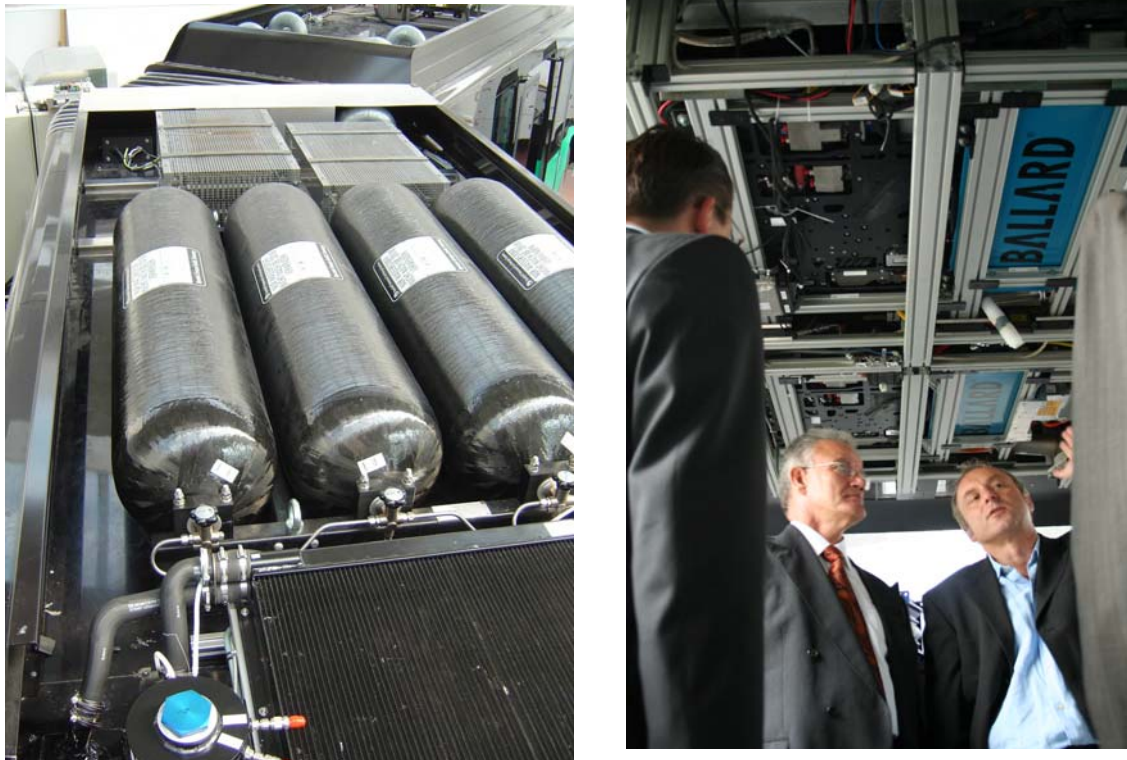
Figure 29: H 2 storages and PEFC twin cluster installed under the roof of the AutoTram
