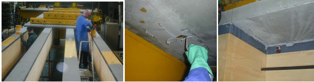
Figure 7 : Glue application on the beams and the slabs after surface preparation (rubbing down)
