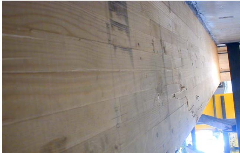
Figure 18 : Tensile (vertical) cracking in the mid-span zone for beam P2
