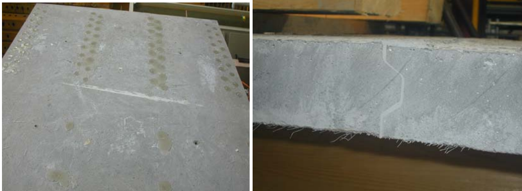
Figure 8 : Details. Left : filled reservations over the long screws. Right : joint between slabs (after sawing of the model)
