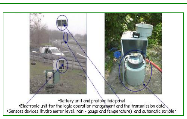
Figure 10 Water pollutant monitoring system instrumentation on motorway A7
