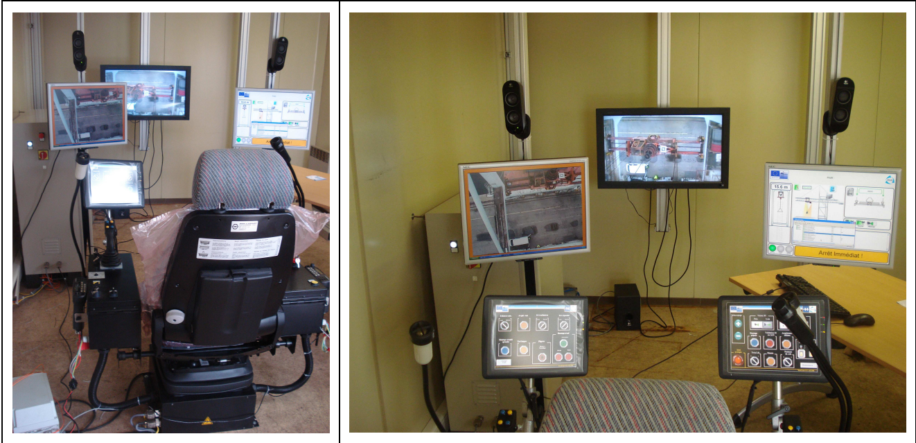
Figure 2: SECURCRANE Remote Control cabin (with integrated Anti-Sway Module)
