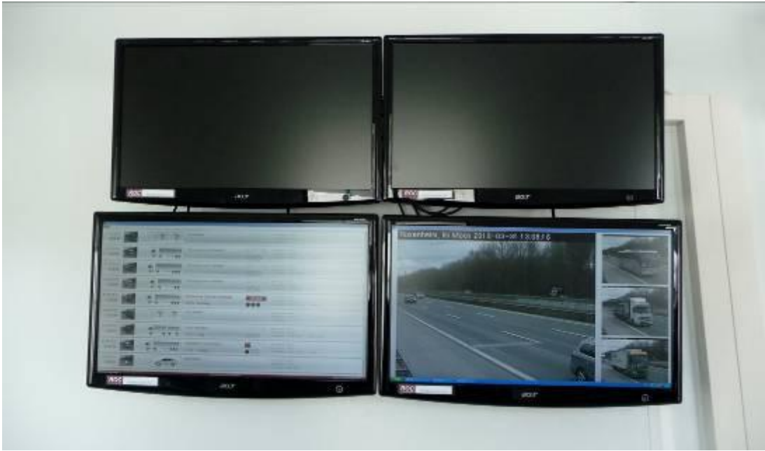
Figure 41: Installation of the high-resolution traffic monitoring system for observing the current situation on the highway.
