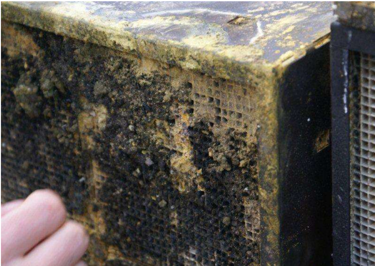
Figure 62: SCR element clogged by particles
