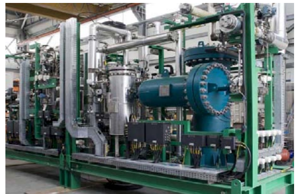
Figure 2: On-site reformer realised in Mantova
