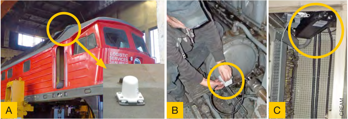
Figure 38: NavMaster LT – Installation of telematics system in Romania. A: Roof mount GPS/GSM antenna. B: Installation of electronic fuel tank sensor. C: NavMaster LT in electrical cabinet
