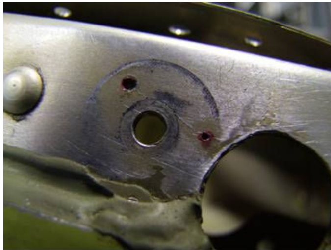
Figure 191: Detailed view of a crack next to a rivet hole
