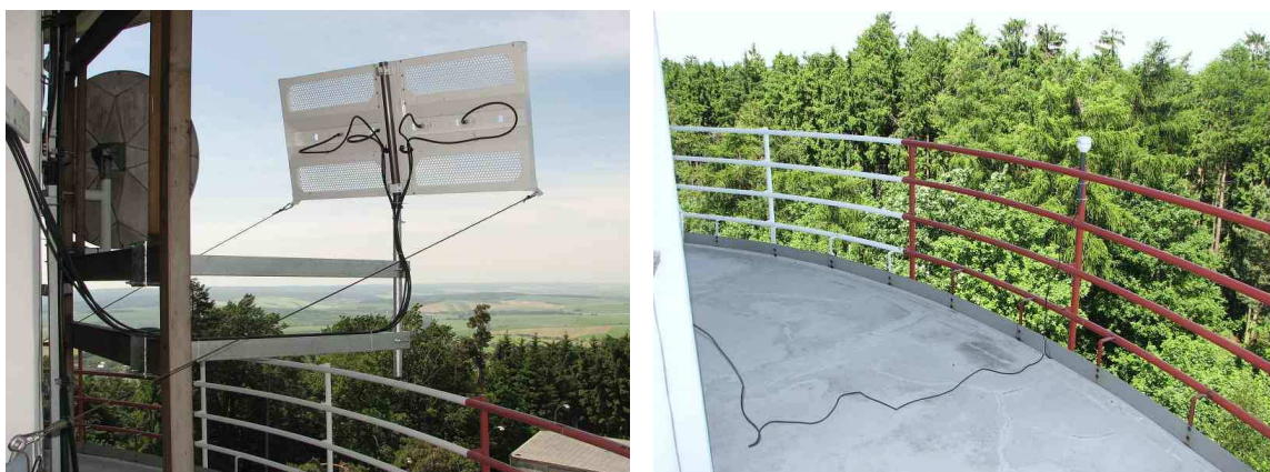
Figure 13. Hradisko installation, PCL and GPS antennas.
