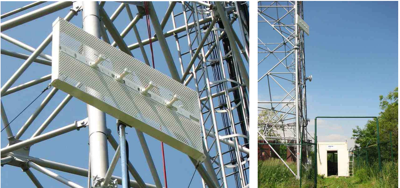
Figure 14. Kadovska Hora installation, PCL antenna.
