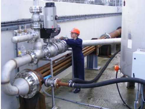
Argon Supply System: Boiler (most remote from camera), Superheater, flow control valves. The 5tonne water supply tank is extreme right of picture.
