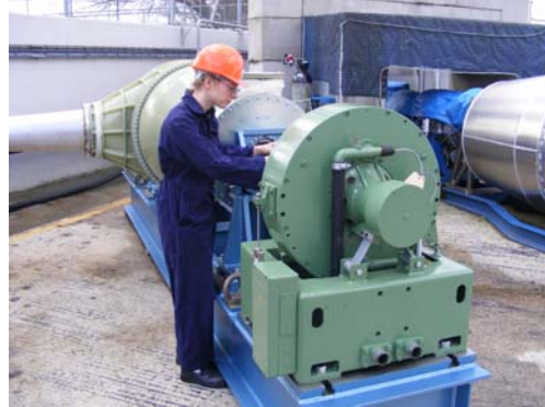
Turbine and one of the two dynamometers. The argon inlet diffuser enters from the left of the picture.
