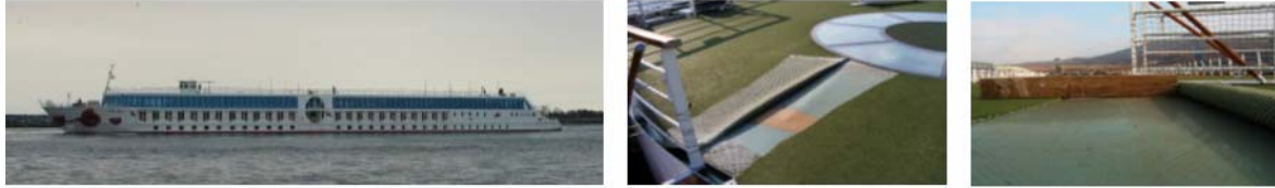
Figure 6.2.1-2 - all-metal sandwich repair case study. Left: AROSA river cruiser. Centre: damaged area. Right: buckle in the sun deck.
