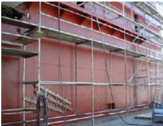
Figure 2.3-1 - funnel casing with improved thermal insulation (SPS – steel facings and polyurethane elastomer core).
