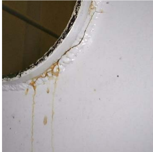
Figure 6.1.1.2–2 - corrosion streaks developed by a sandwich panel in service.
