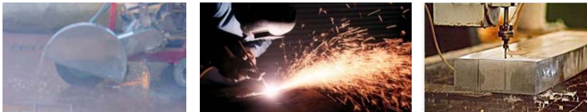
Figure 6.2.2-1 - from left to right: cold cutting of an SPS panel, air carbon arc gouging of an SPS panel, and water jet cutting of an SPS panel.
