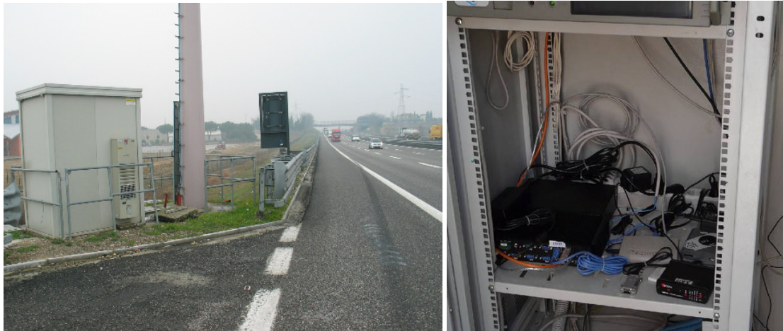
Figure 34: Shelter box hosting the RSU system devices
