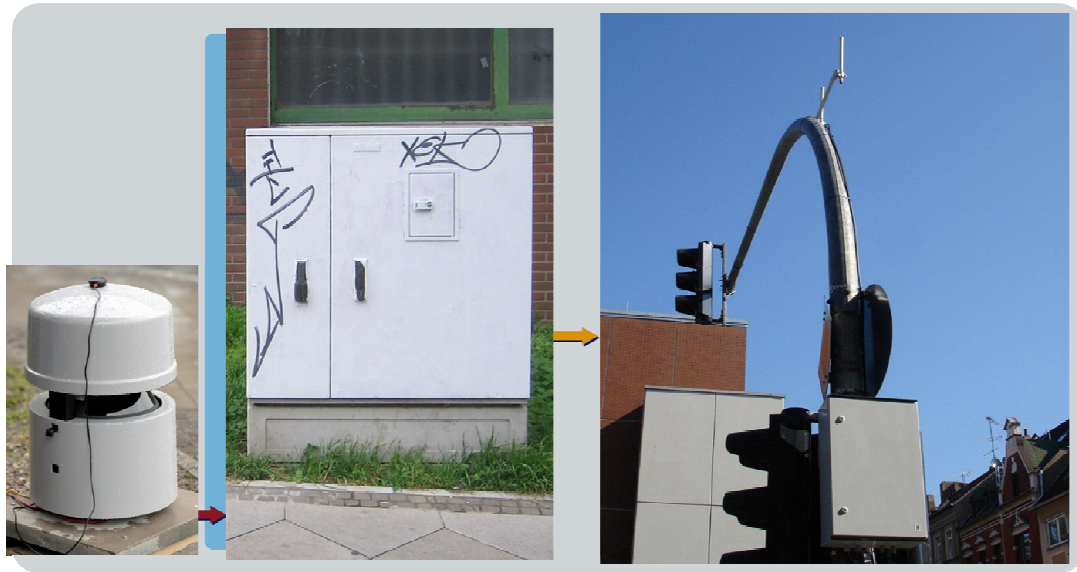
Figure 48: Equipment installed in the Dortmund Test Site
