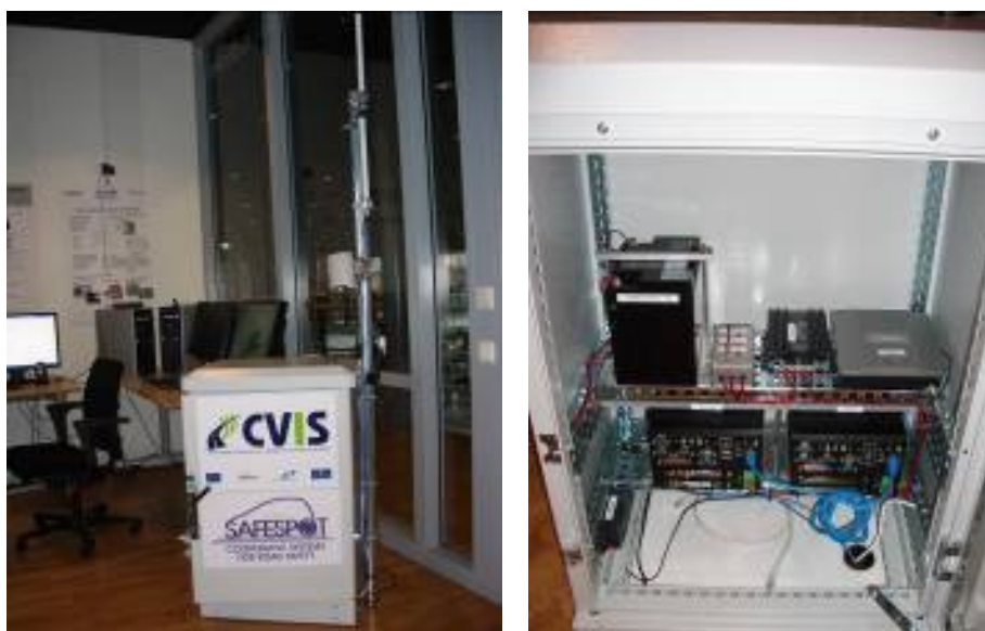
Figure 70: Mobile RSU installation (Main PC, Router, 3G Gateway and internal power supply)
