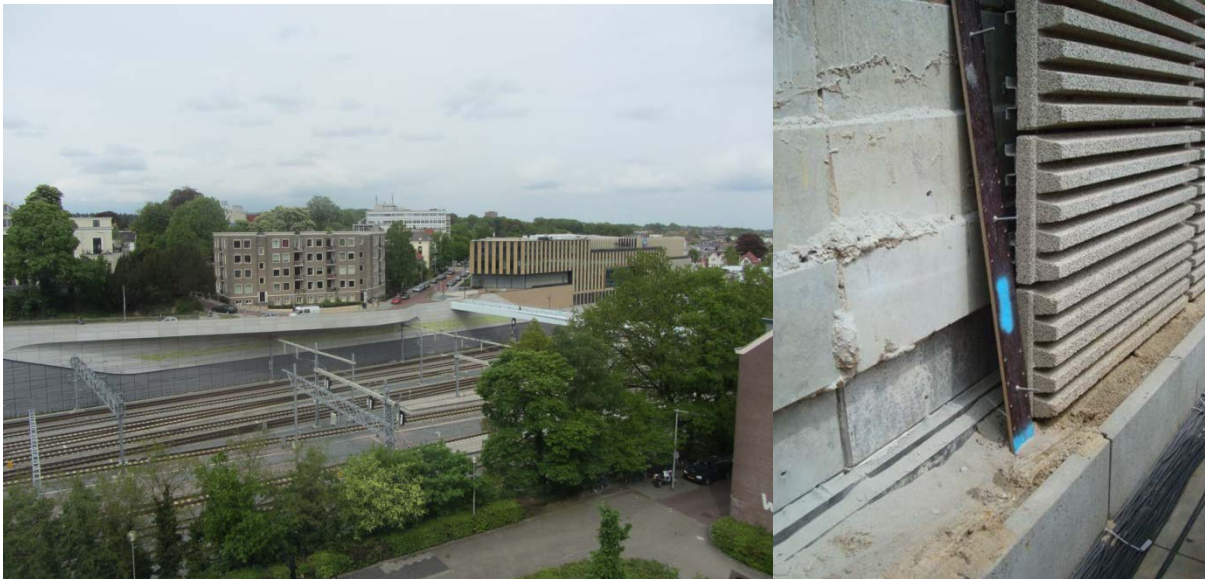
fig. 12: coated ground wall, built in Arnhem, The Netherlands; in the left picture the top of the resilient layer can be seen (two 60 mm black slabs, partially covered with sand), just where the ground wall surfaces and continues as a ground retaining wall (with sound absorbing panels)
