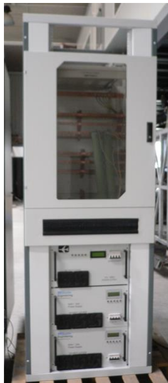
Figure 2. PTB Electrical Cabinet
