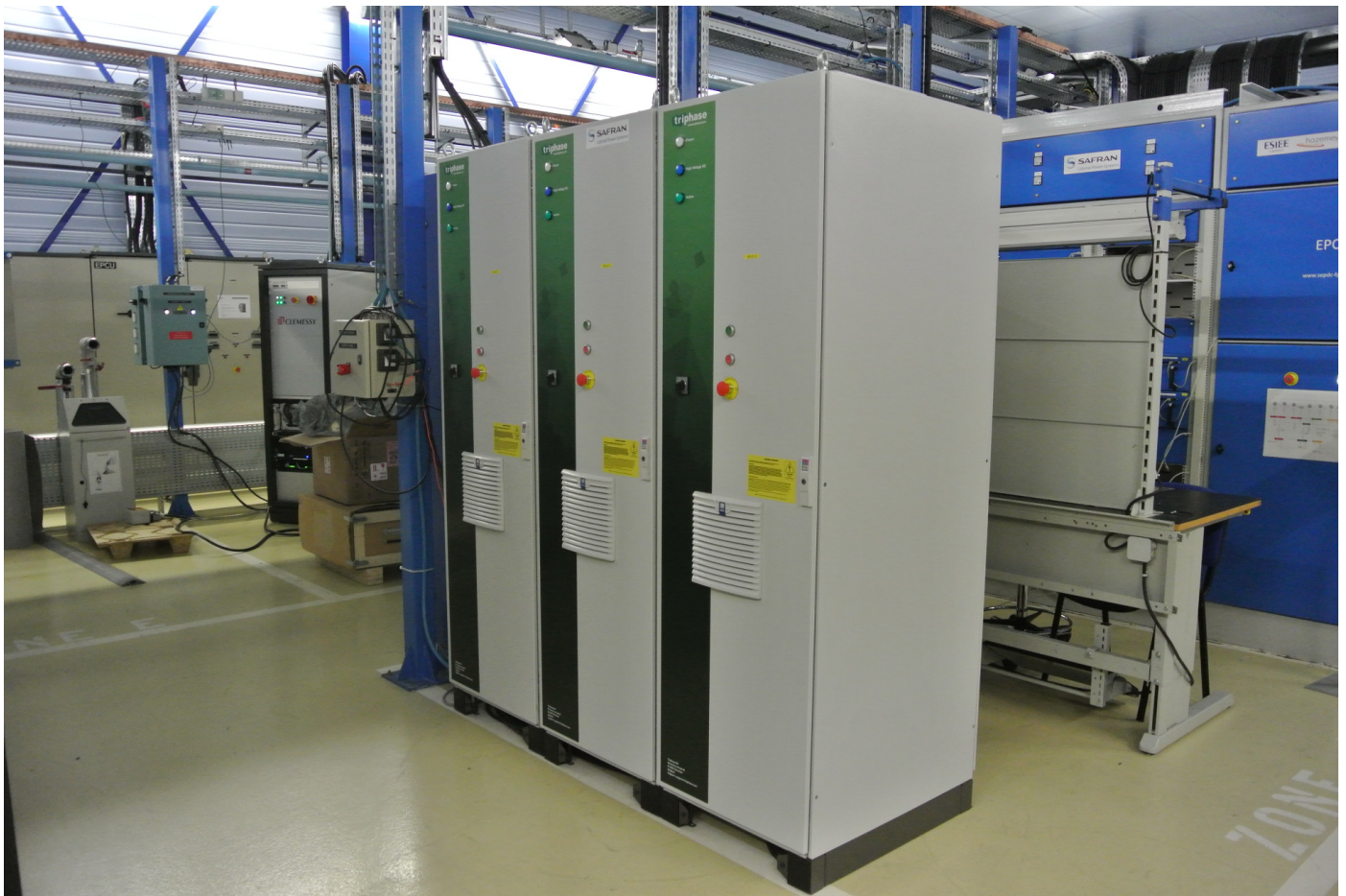
The SPLS modules in place at the Clean Sky lab.
