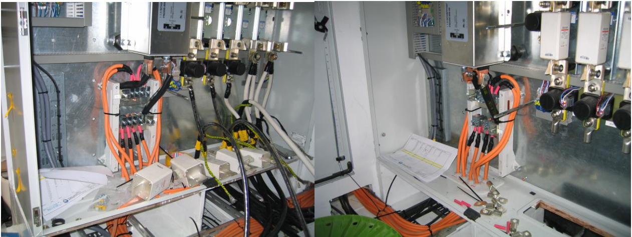
Illustrations: More installation work: From inside port side cabinet (left) and SB side cabinet (right).
