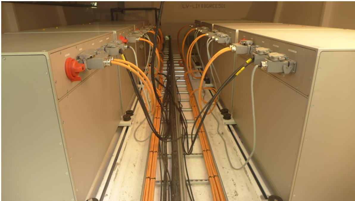
Illustration: The battery modules manoeuvred on place inside the BB GREEN test vessel connected and successfully tested. Each module unit has a weight of approx. 450 kg.
