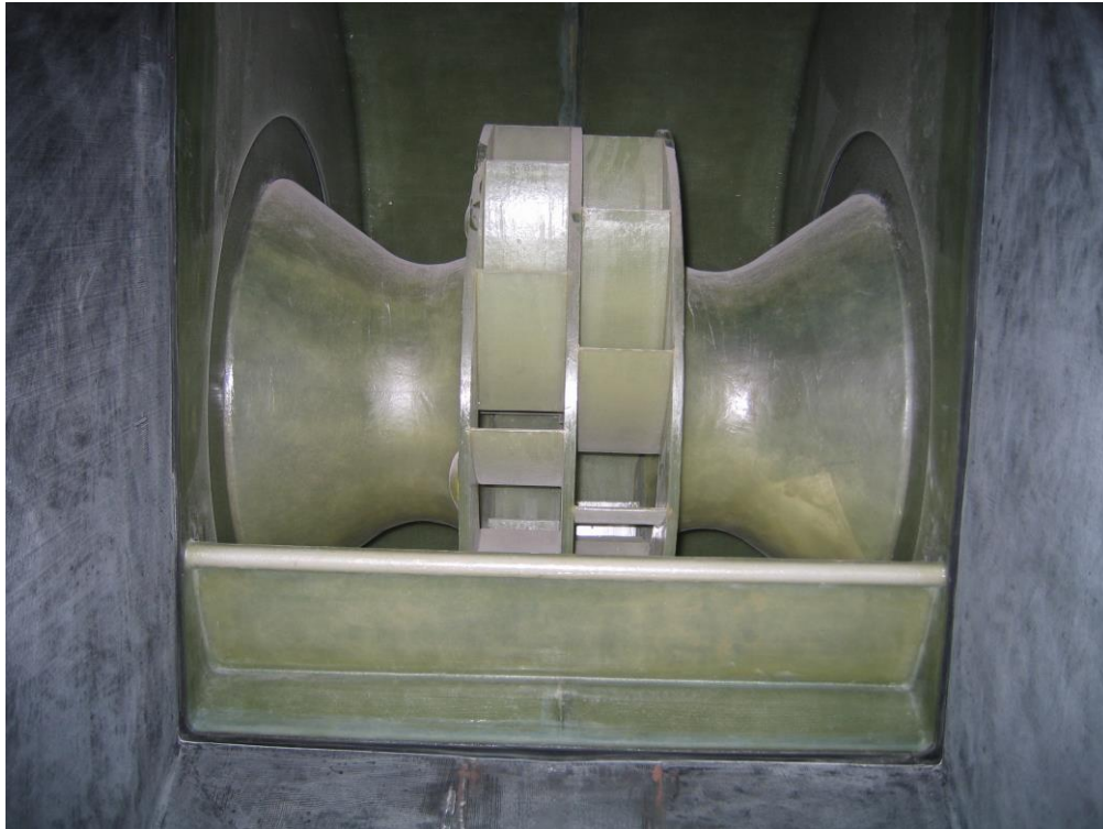
Illustration: Picture from inside the air channel up towards the lift fan impellers.
