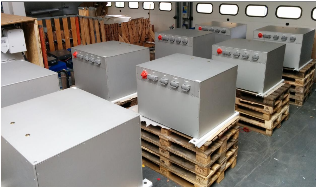
Illustration: Battery test set up prior to shipment to the yard for installation.
