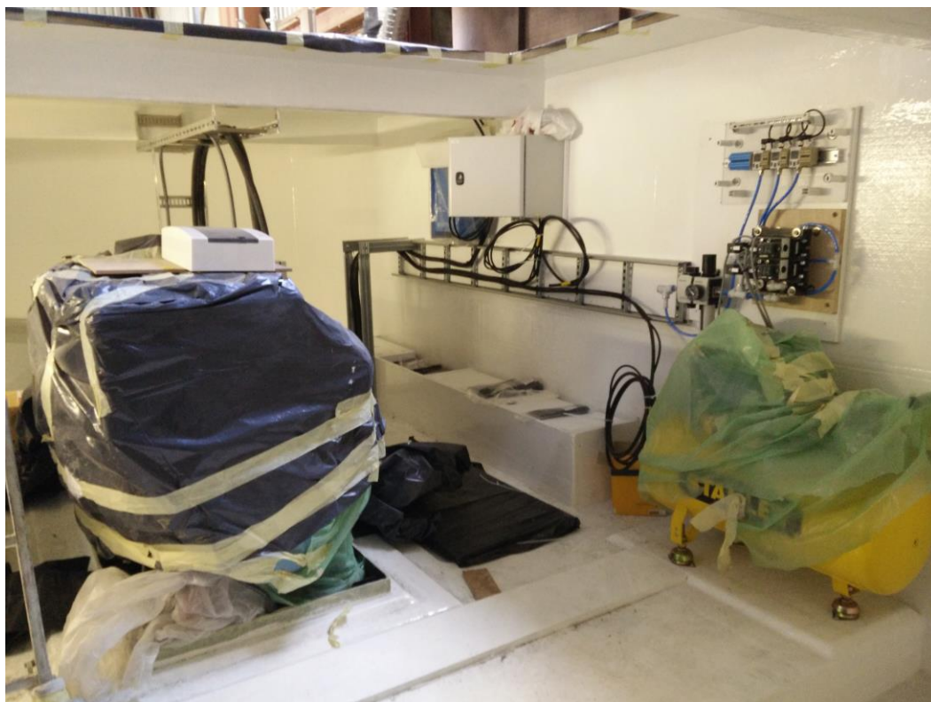
Illustration: More installation work, from installation of generator set / range extender (wrapped in - left) and mounting of ASV control / flap system elements (yellow compressor wrapped in plastic to the right).
