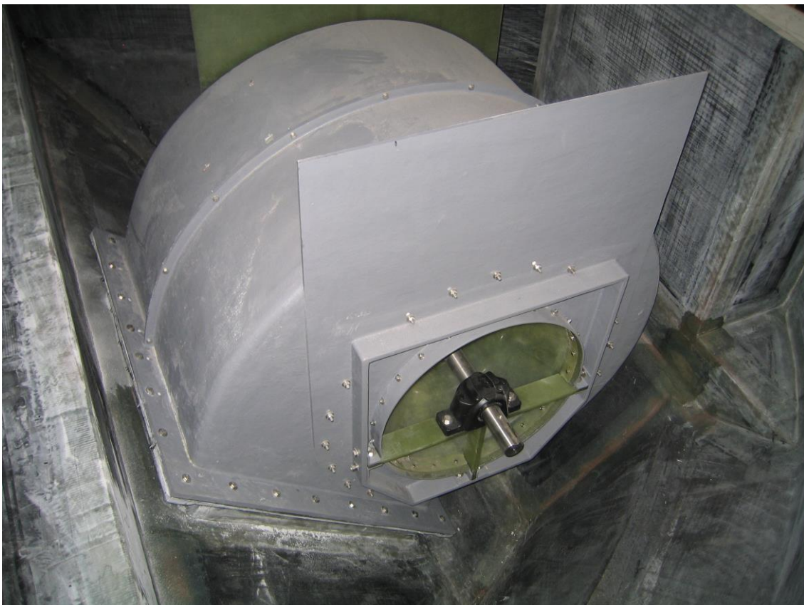
Illustration: Lift fan installed in the lift fan room forward, ready for priming and sound damping.
