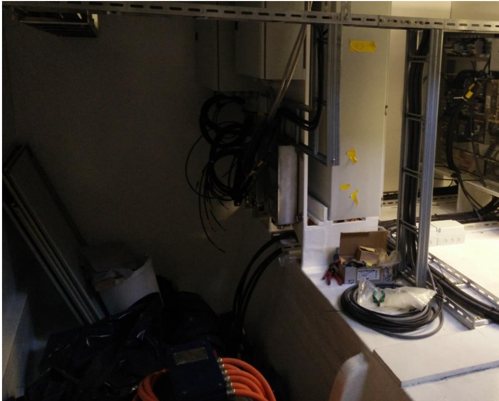
Illustration: From mounting of the electric driveline in the BB GREEN propulsion gondola.
