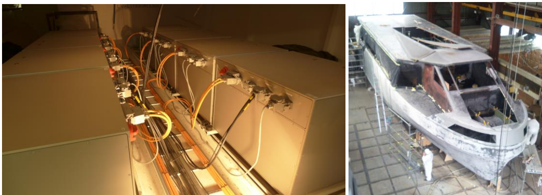
Illustration: Battery bank installed & tested inside the test vessel. From construction. (right).
