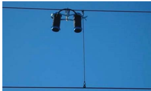
Figure 1 – On-line camera from OH-line for measurements in S&C
