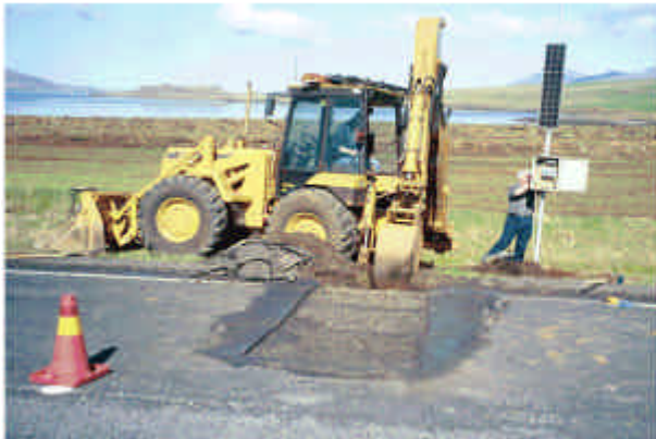
e) Datalogger and Solar Cell Mast and Instrumented Pit after Compaction of Unbound Layers
