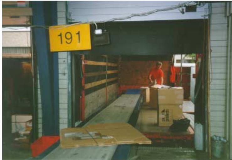
Figure 13: Automatic transportation belt reaching inside the “loading gangway”
